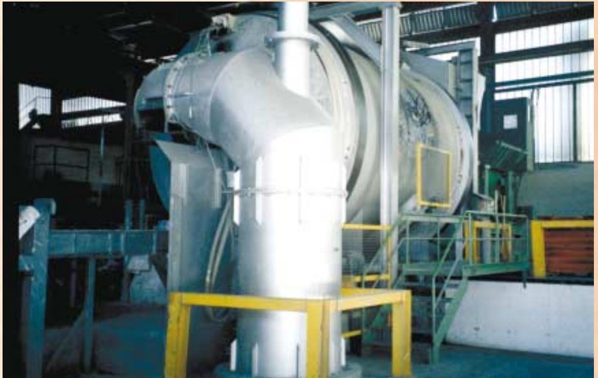
Integrated burner block and exhaust system for double pass operation
